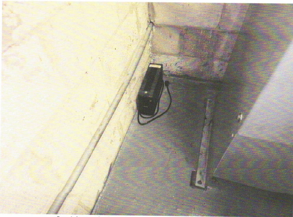
Repair battery backup system at Building 8 for proper operation
