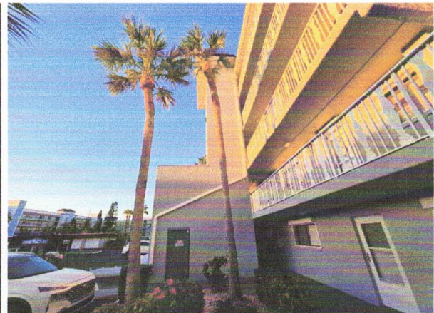
Hoistways located outside, recommend pit sump pumps
