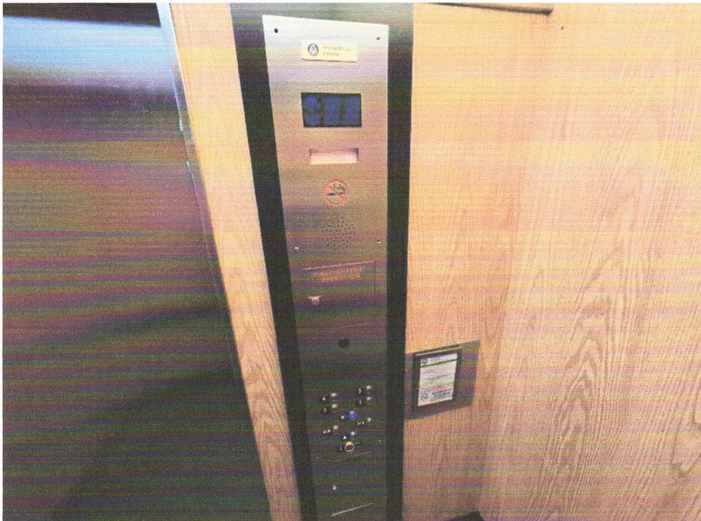
Repair position indicator in Car Operating Panel at Building 9
