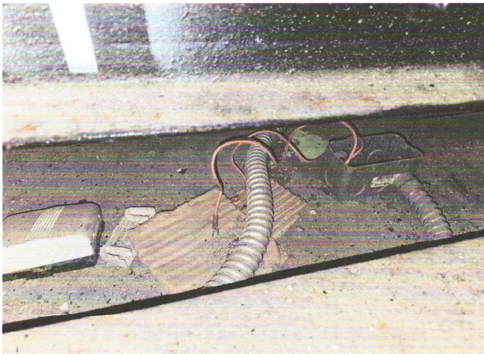
Properly insulate exposed wiring & reinstall junction box cover on car top at Building 9
