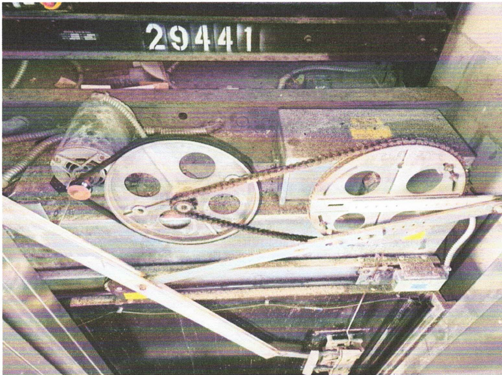
Clean car top. Clean, lubricate and adjust door operation system at Building 9
