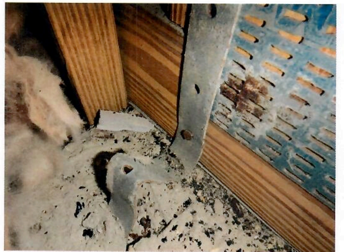
Toe nail (1/2" off truss)
