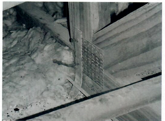
Toe nails (doesn't meet nail requirements)
