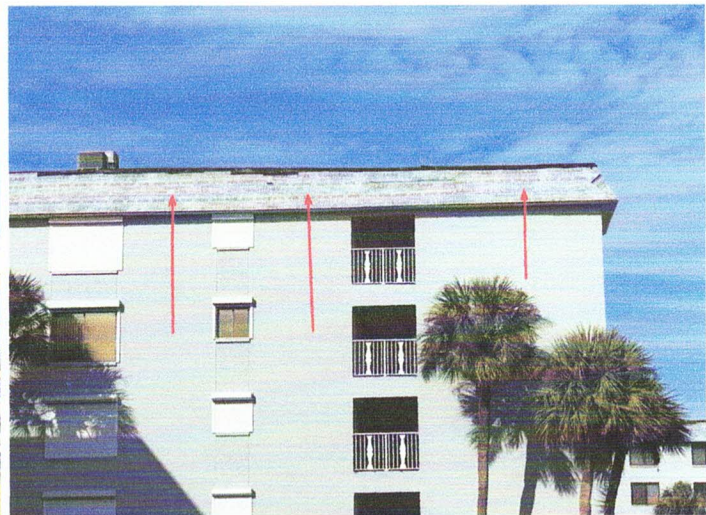
In progress installation of the self-adhering underlayment to the wood decking at conditions of the mansard.
