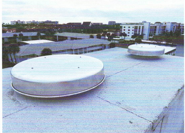
Completed installation of the new roof vents to replace existing on the elevator roof section.
