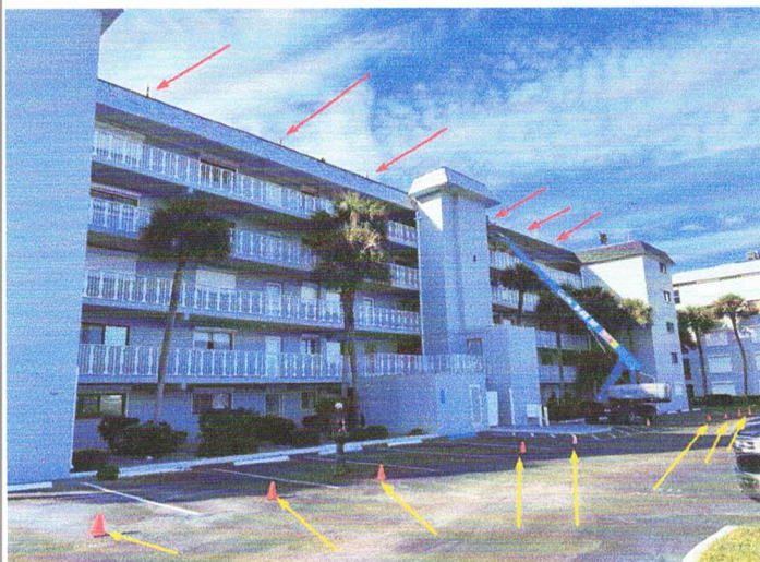
Red arrows indicate roof perimeter warning line system in place. Yellow arrows indicate ground markers or lift procedures.
