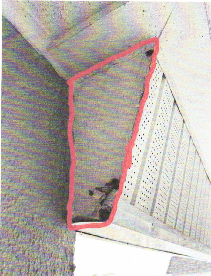
Red highlighted area indicates existing soffit end closure that will be replaced with new.
