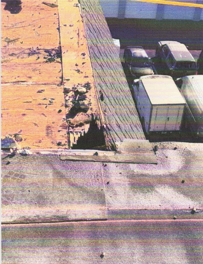
Typical deteriorated wood decking at the perimeter.
