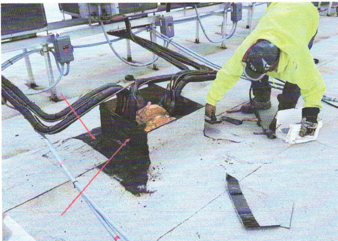
Red arrows indicate torch priming process was used in the flashing procedures.
