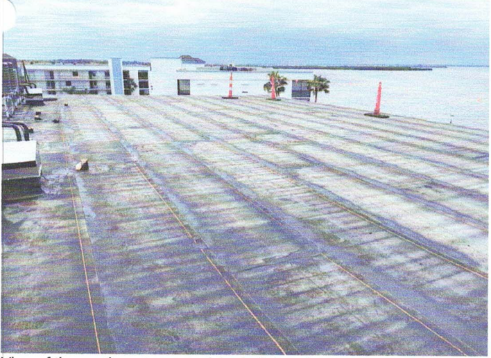
View of the southwest corner of the building after installation of the plywood vapor barrier, 1/8" sloped insulation and modified interply sheet. All laps have been heat-welded to be watertight.
