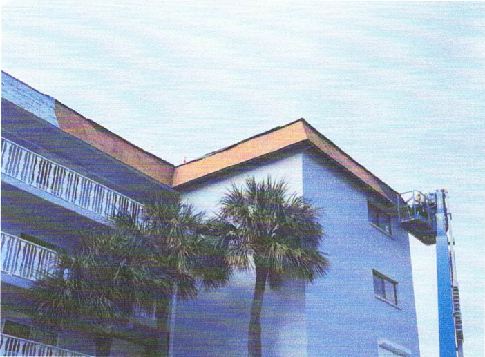
View of the exposed plywood sheathing on the mansard. All wood appears to be in good condition. The existing soffits have been removed and discarded. New vinyl soffits will be installed.
