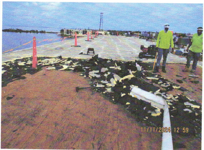
View of the roof removal in the southwest corner of the roof, looking north.
