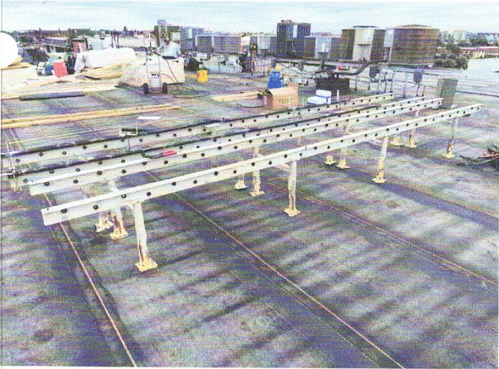
Photo of the old mechanical stands that have been removed and will be disposed of off site.
