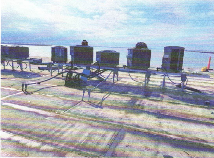
Photo of the new mechanical stands, to include new copper lines, electrical lines, disconnects and hurricane clips.
