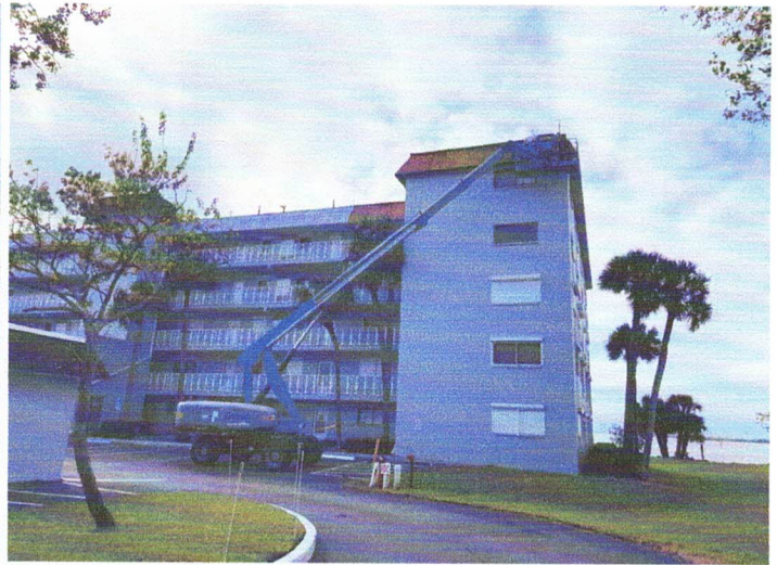
Tech System roofers removing the existing shingles, and installing new self-adhered roof underlayment on Bldg #9.
