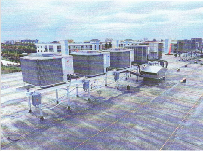
Photo showing the newly installed aluminum mechanical stands, with new copper lines, insulation, electrical whips, electrical conduits, hurricane clips and new stainless-steel mechanical chase cover.
