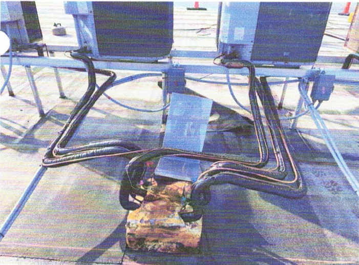
Close up view of the new mechanical lines with new insulation. A stainless steel chase box will be installed over the chase during final roofing detailing.
