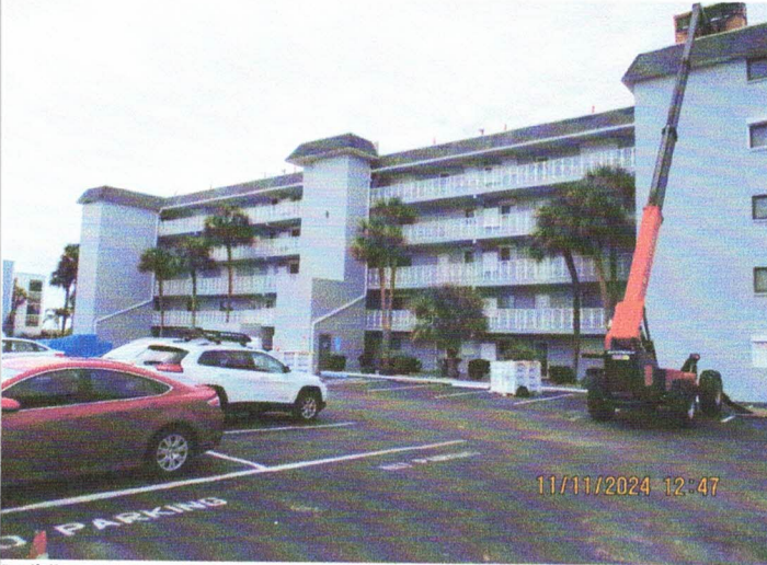
Building #8 re-roof was started on November 11th. Safety flags are staged around the roof perimeter with trash being downloaded in a impbox attached to the lull.
