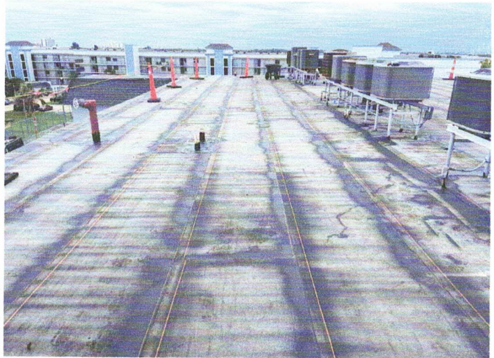
Another view of the roof installation looking south. New mechanical stands have been installed by Erwin Air. After all work is completed the final granulated cap sheet will be installed as the finished roof surface.
