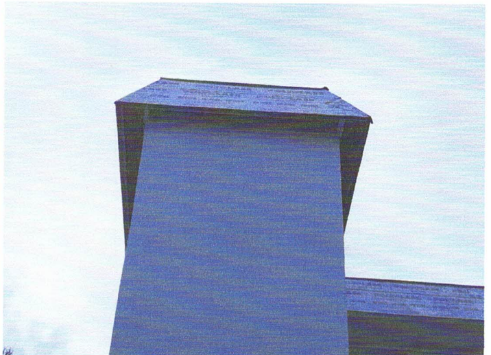
View of the south side mansard on Bldg #9, with soffits removed and new underlayment installed.
