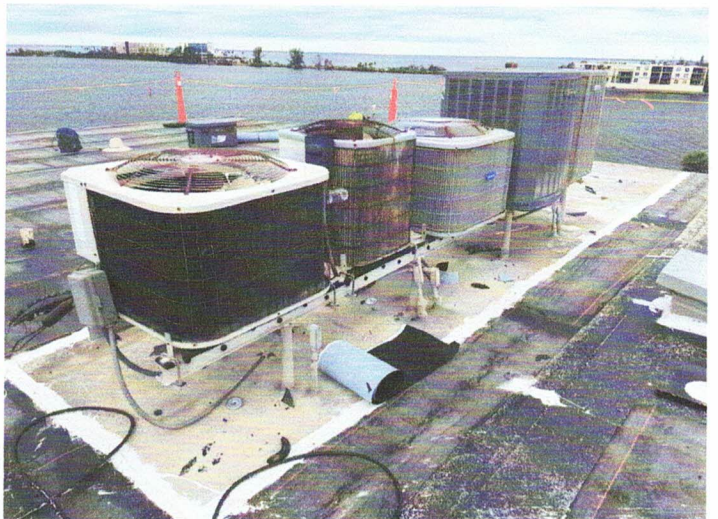
There is one final group of a/c condensers that will be disconnected on the north side of Bldg #8.
