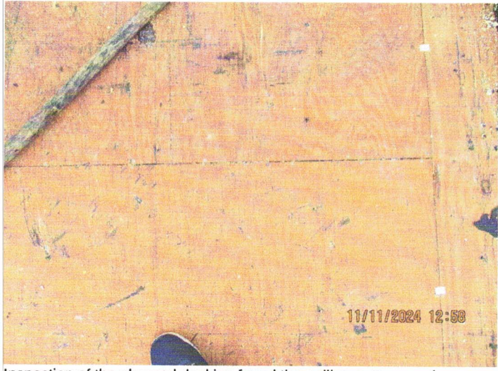
Inspection of the plywood decking found the nailing pattern on the plywood ends to be code compliant at 6" on-center or more. However, the trusses located in the center of the plywood only have roofing staples. Tech System is adding roofing nails at 6" on-center to the center of the board located over trusses.
