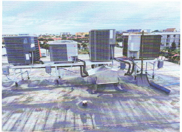
Another view of completed a/c condenser stands. Note that the new stands are longer to for proper spacing of the larger condensers for proper air flow.
