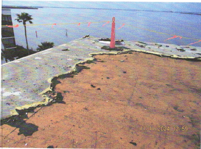
View of roofing being removed from the southwest corner of the building. Existing roof is a spray polyurethane foam roof over an existing modified roof on a plywood roof deck. This section of roof decking is in good condition with no deterioration noted.
