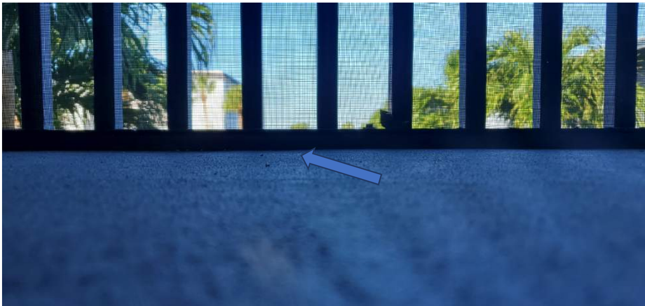
Example view of no shims under screen which prevents positive drainage
