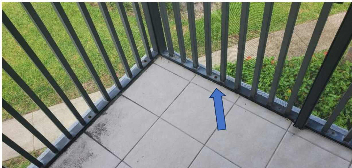
Example view of rusting screen fasteners and tiled concrete slab
