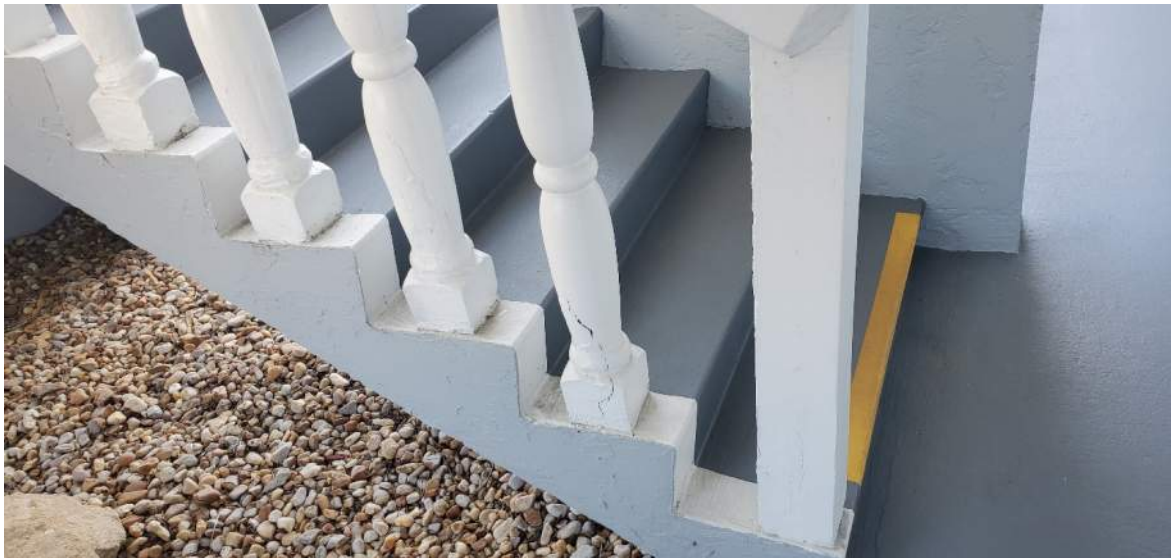
Example view of spalling concrete stairs post
