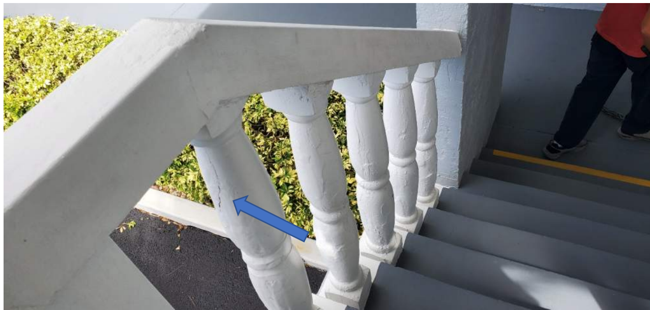
Example view of concrete walkway stair railing pickets spalling
