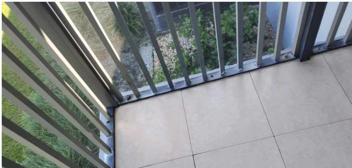
Example view of corroding screen railing fasteners
