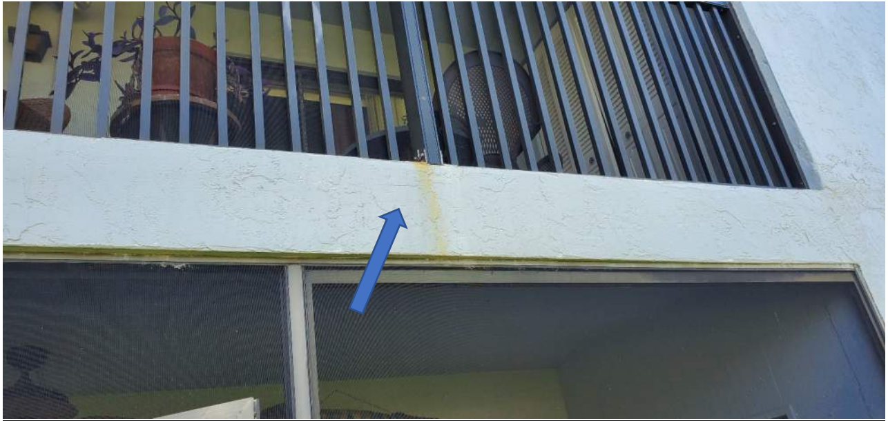
Example view of rust stains coming from screen posts
