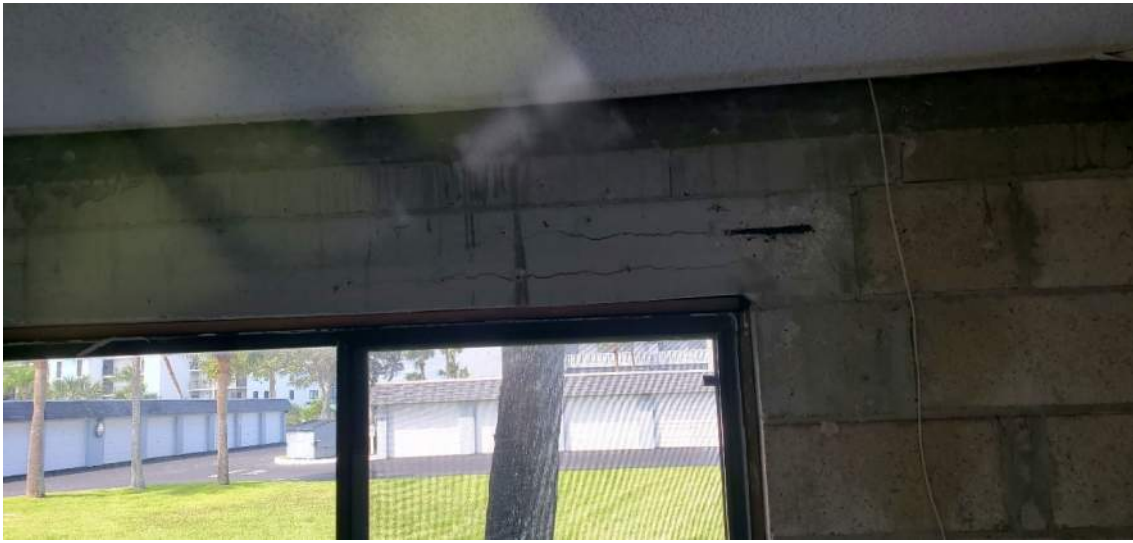
Example view of concrete Header beam spalling
