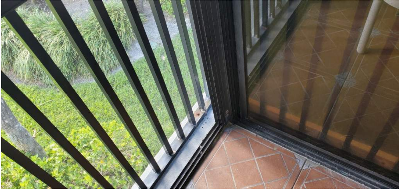
Example view of rusting railing fastener. Note there is tile on the balcony surface.
