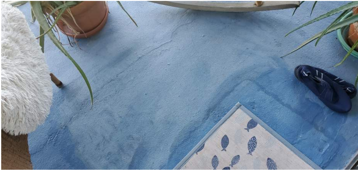
Example view of poor floor coatings
