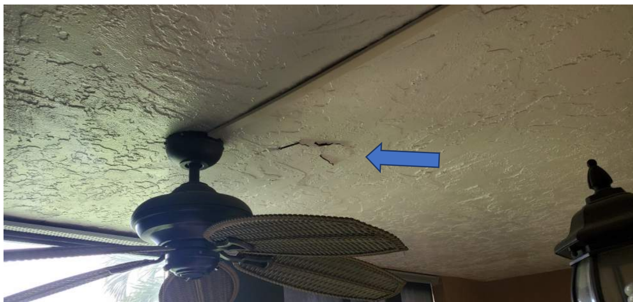
Example view of concrete ceiling spall
