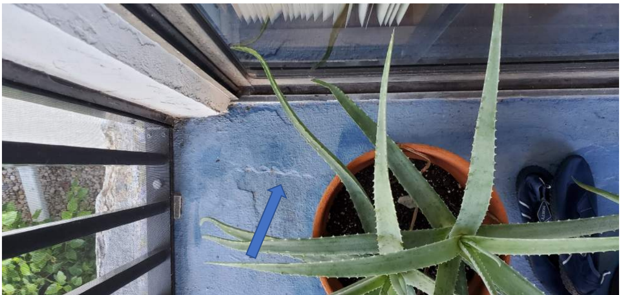
Example view of spalled concrete surface due to corroding reinforcing bars
