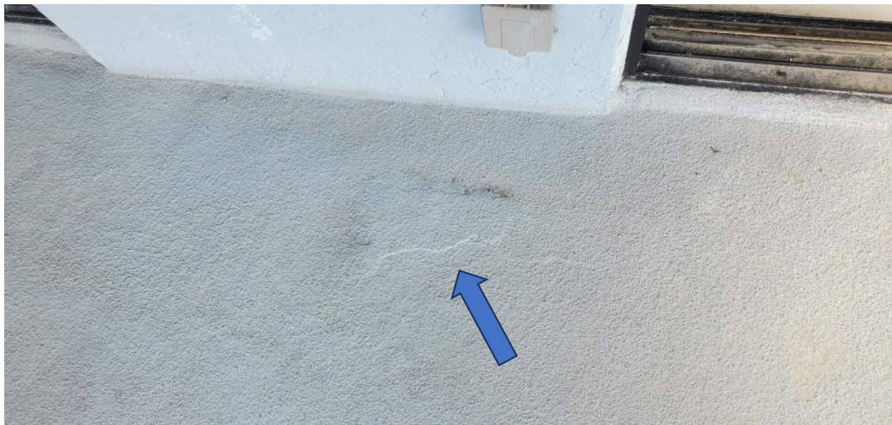
Example view of spalling concrete due to corroding reinforcing bars
