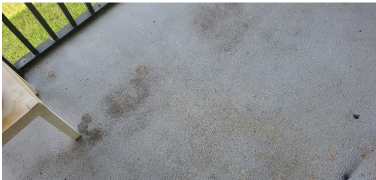
Example view of slab with bad coatings
