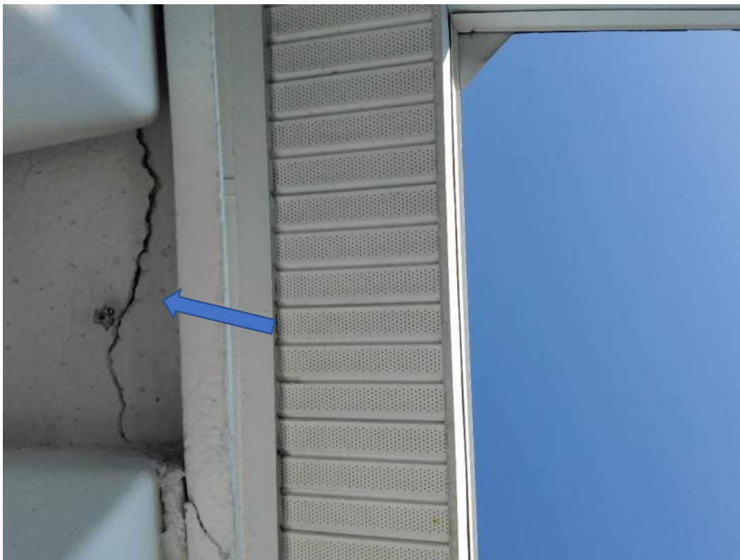
Example view of concrete ceiling spalling
