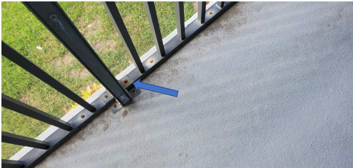
Example view of rusting railing fasteners and worn slab coatings
