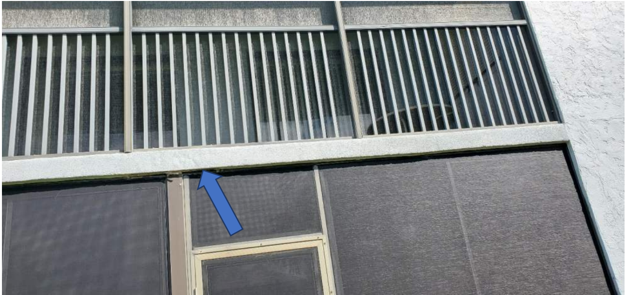
Example view of concrete slab edge spalling
