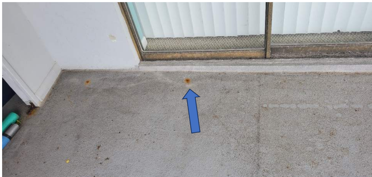
Example view of concrete spalling and rust spots
