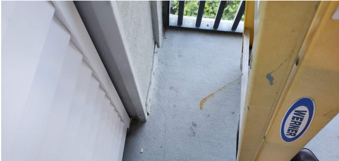
Example view of concrete cracks
