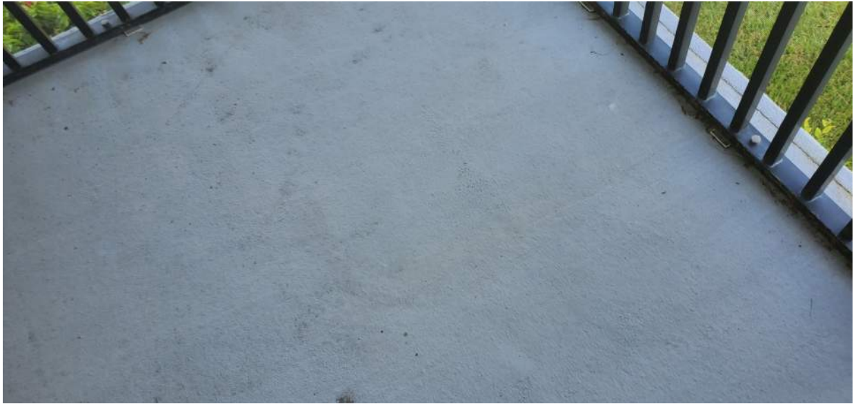
Example view of weathered coating system
