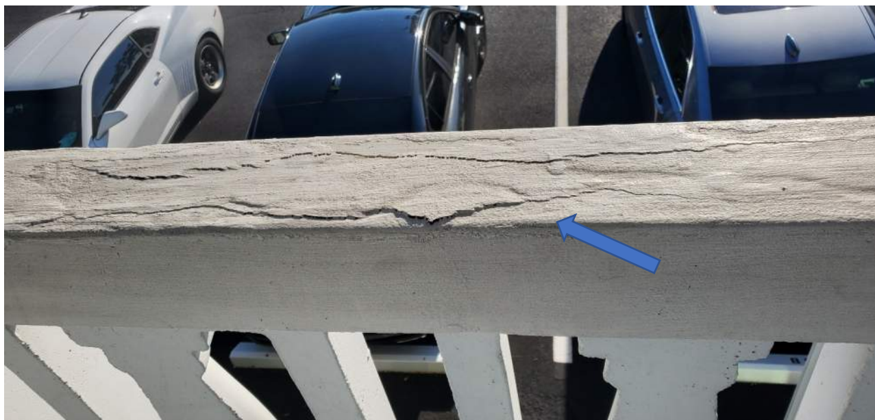
Example view of concrete walkway railing spalling
