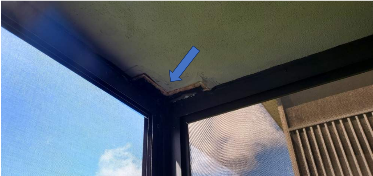
Example view of rusting bearing plate on top of column
