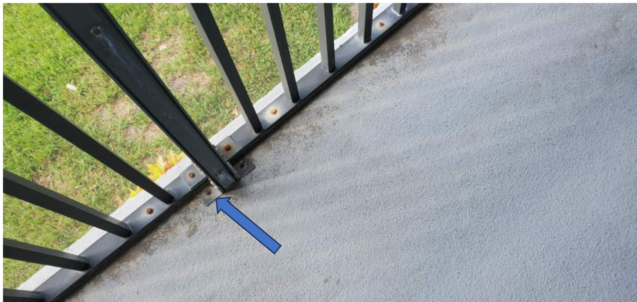
Example view of rusting screen railing fasteners and bad coatings.
