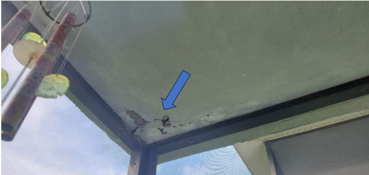
Example view of concrete ceiling spalling
