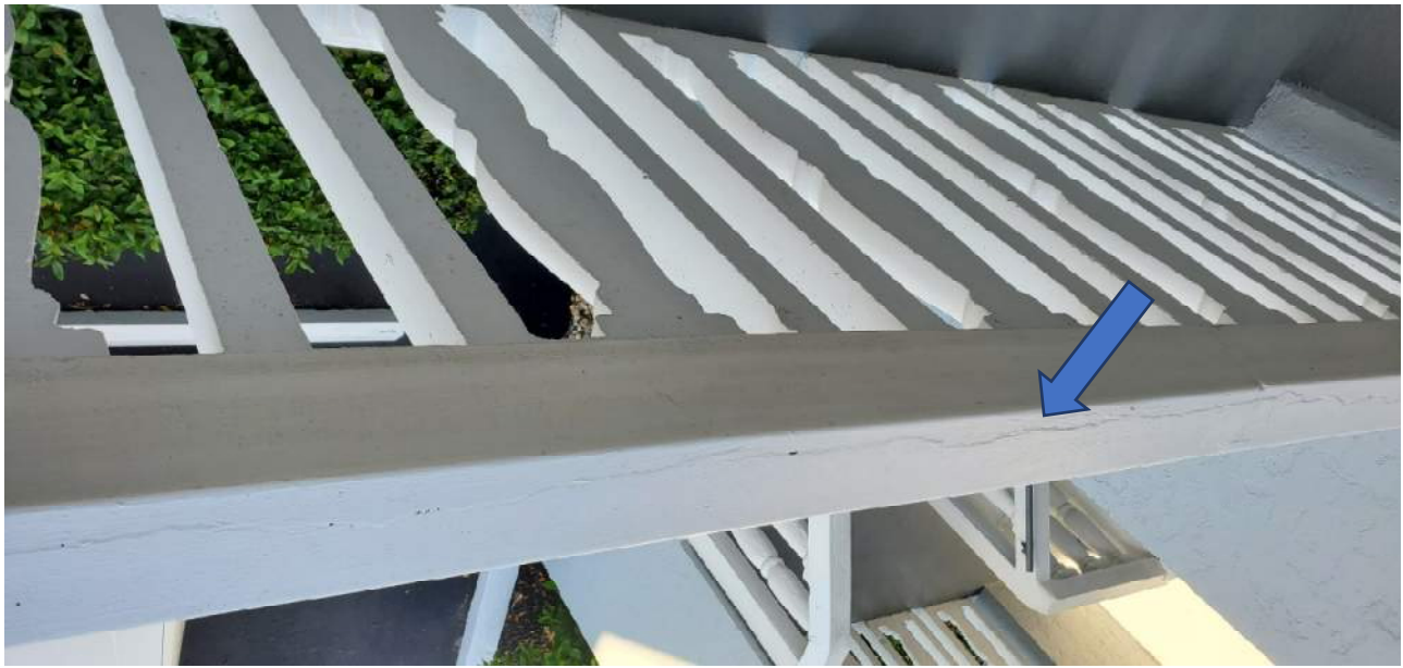
Example view of concrete walkway railing spalling
