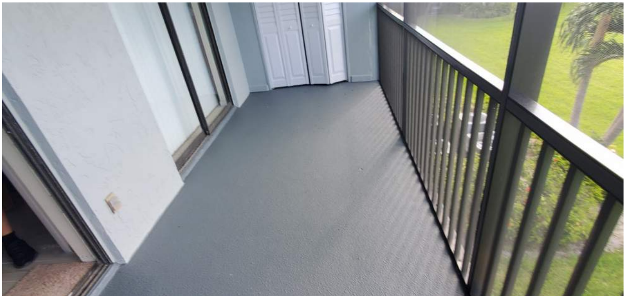
Example view of unit 208. This slab was torn off about a year ago and a new slab was formed and poured with complete new waterproofing coatings.
