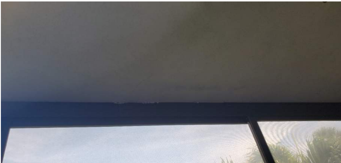
Example view of concrete ceiling staining
