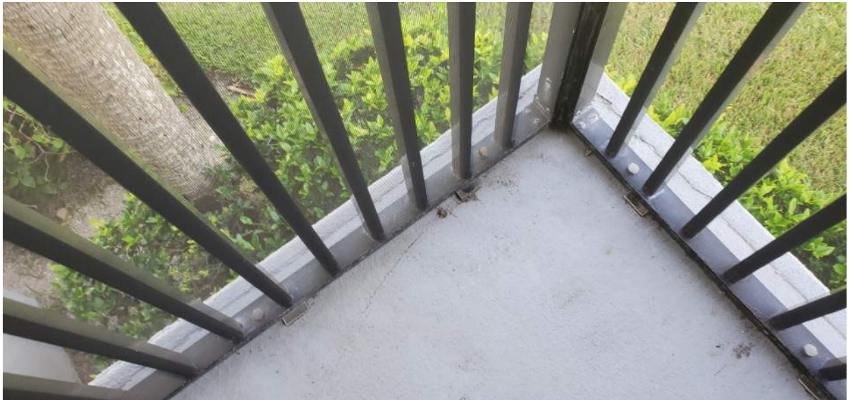
Example view of slab edge spalls
