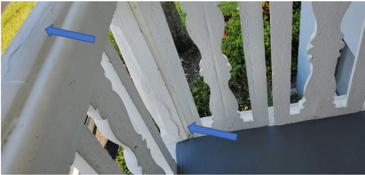
Example view of spalling concrete railings
