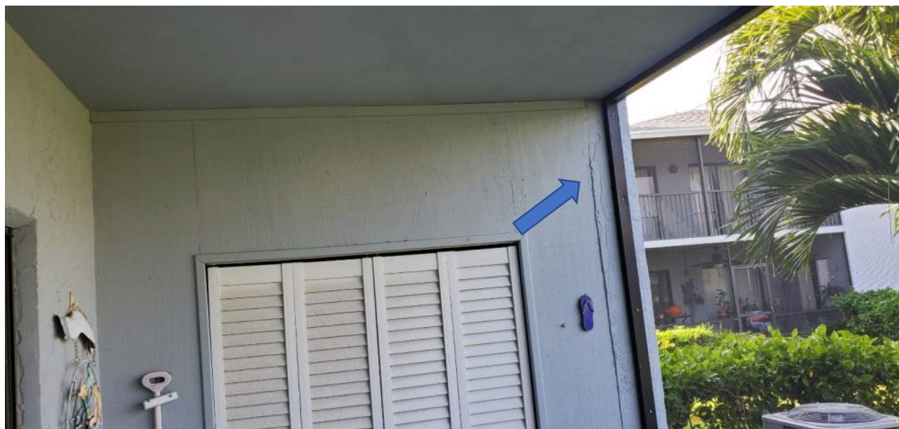
Example view of concrete column spall
