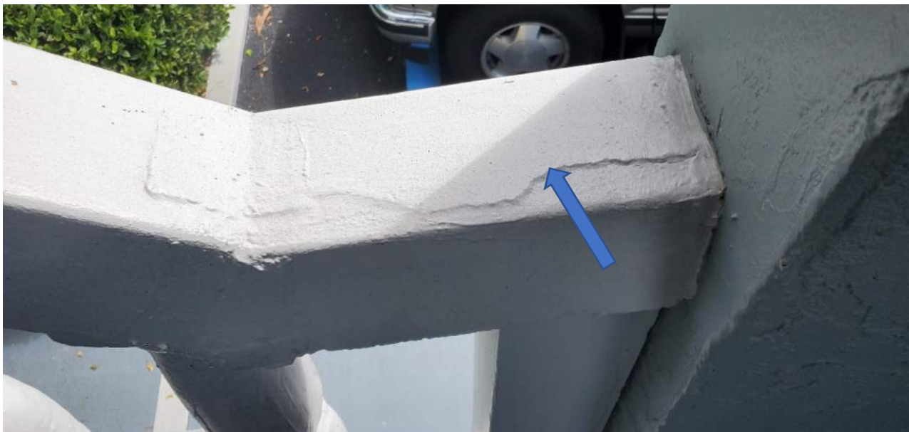
Example view of concrete walkway stair railing spalling
