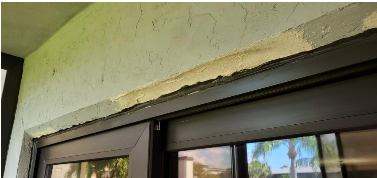
Example view of damaged header that has been previously patched
