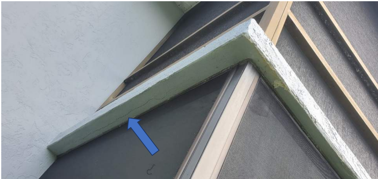
Example view of concrete edge spalling
