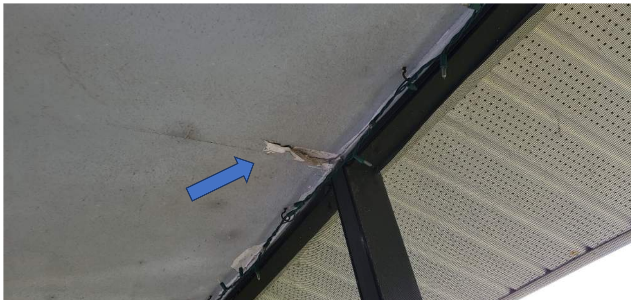
Example view of spalled concrete ceiling
