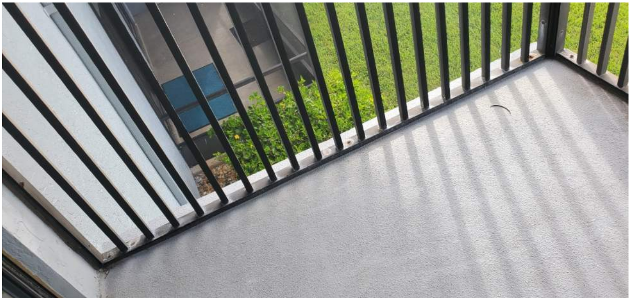
Example view of rusting screen railing fasteners
