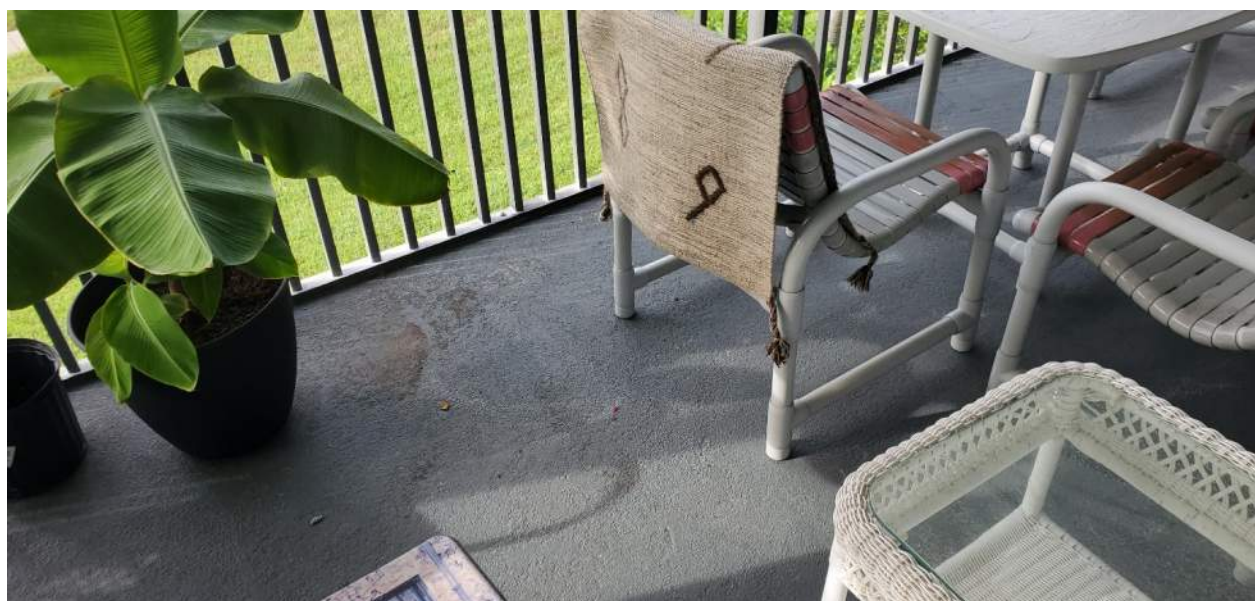
Example view of worn protective coatings
