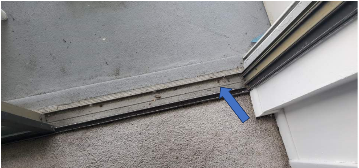
Example view of rusting fasteners at slider
