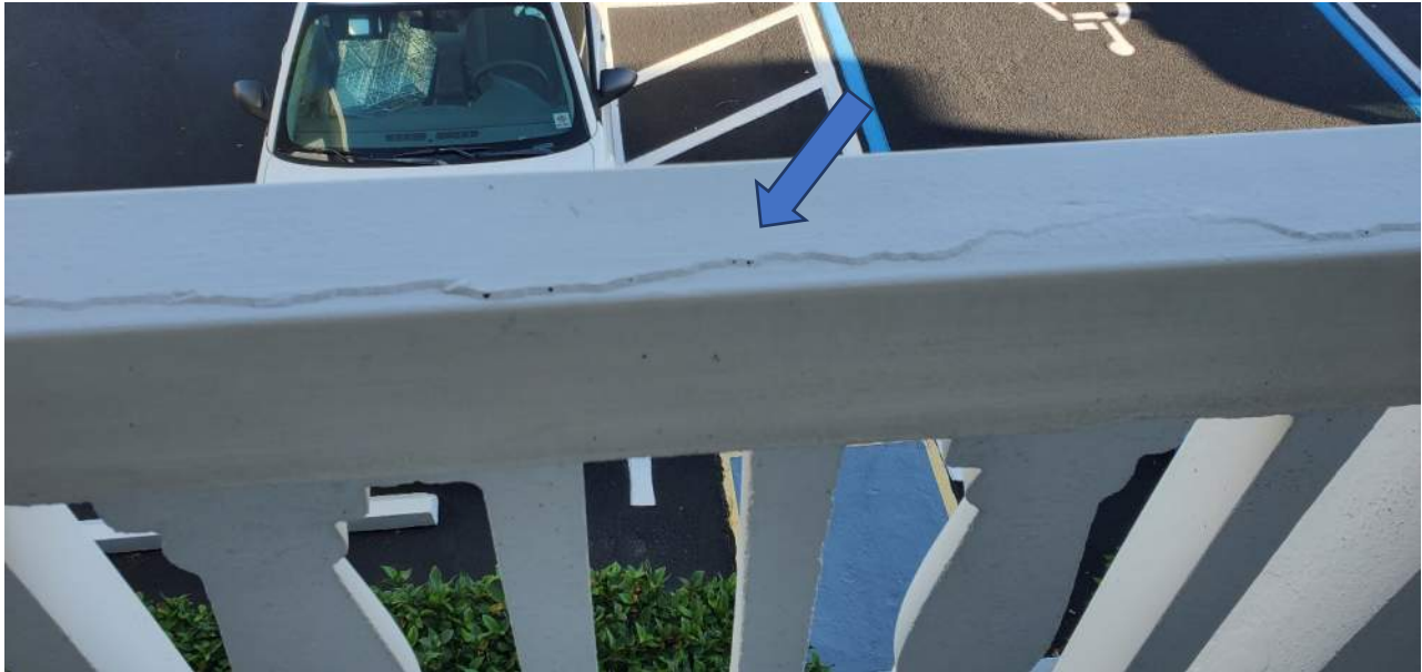
Example view of spalling concrete railings on the walkway
