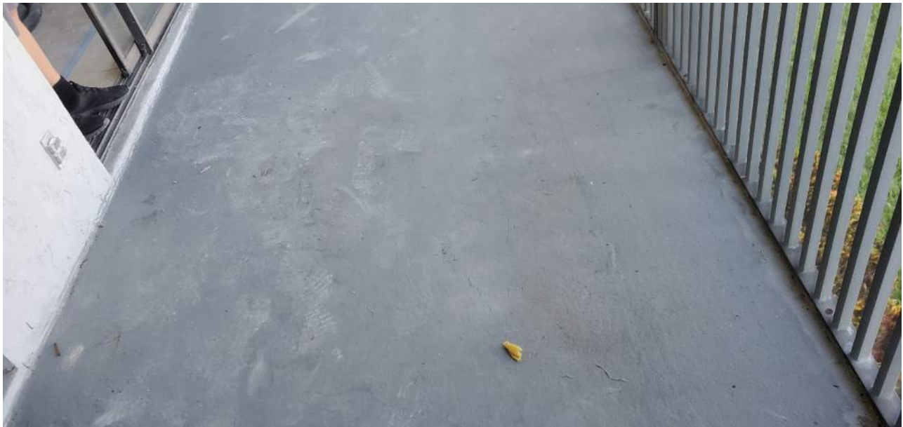
Example view of concrete balcony slab needing new coatings
