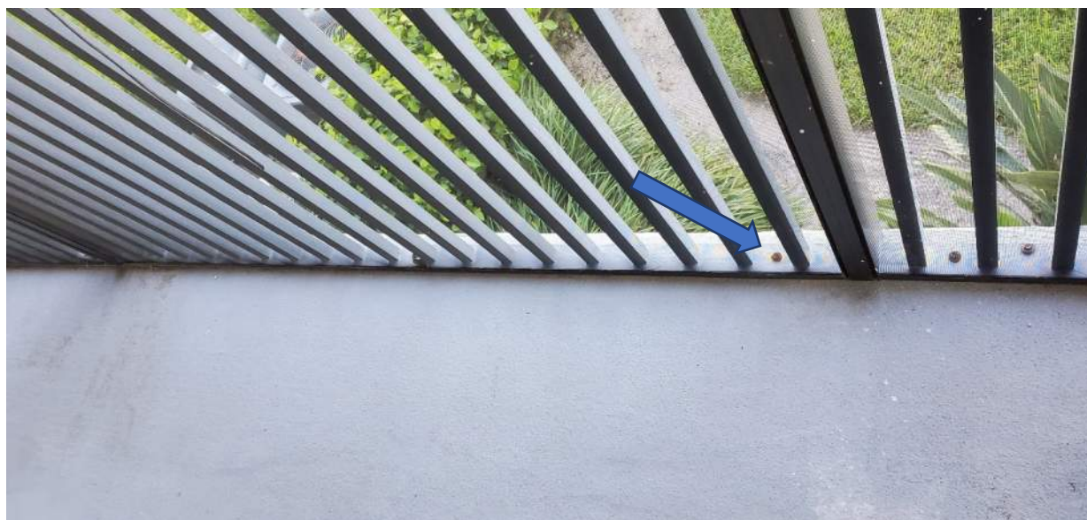
Example view of rusting fasteners of screen railing
