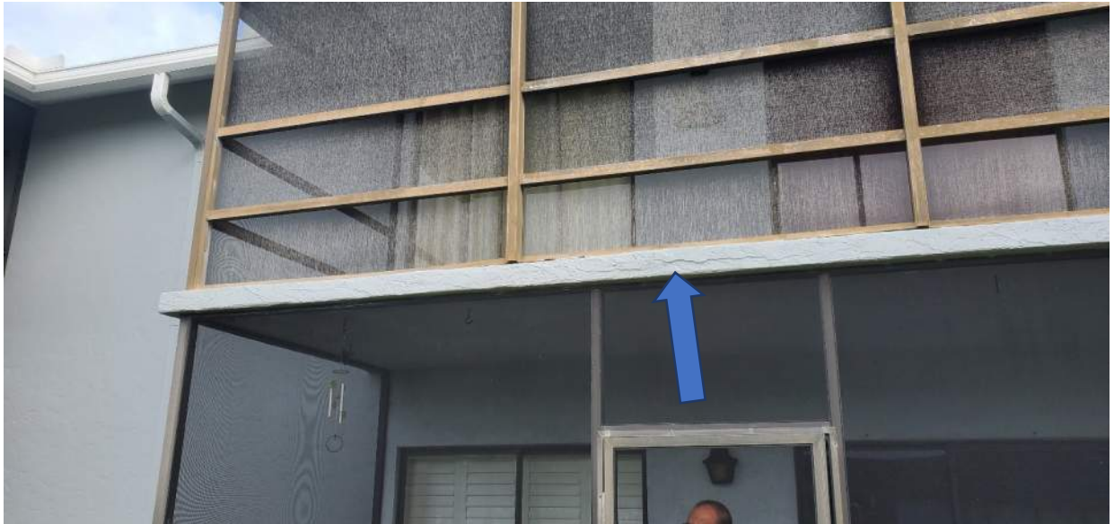
Example view of concrete edge spalling. Note the old style non picket screens
