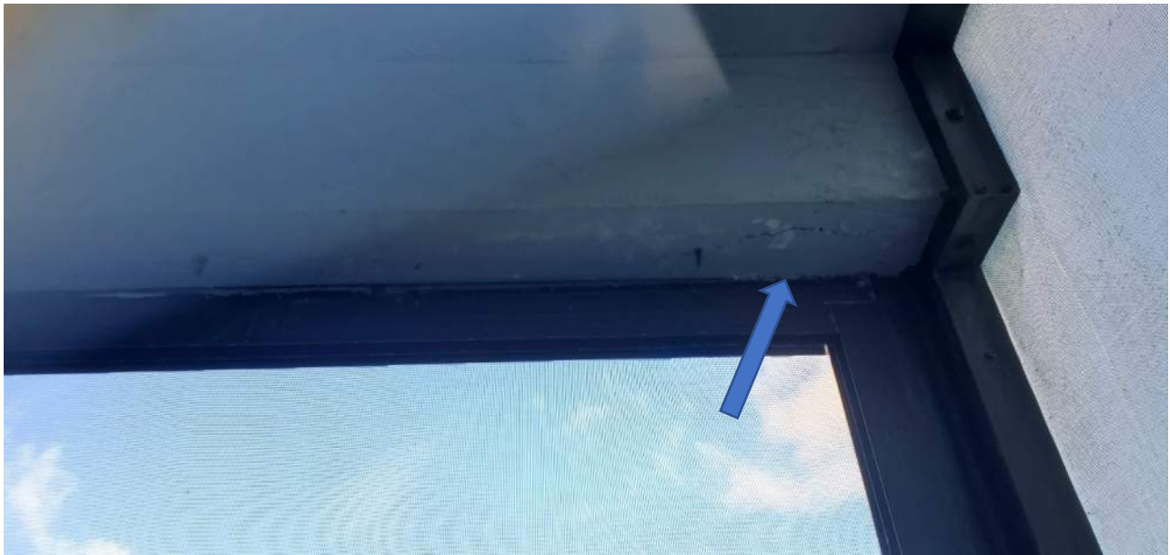
Example view of concrete beam spalling
