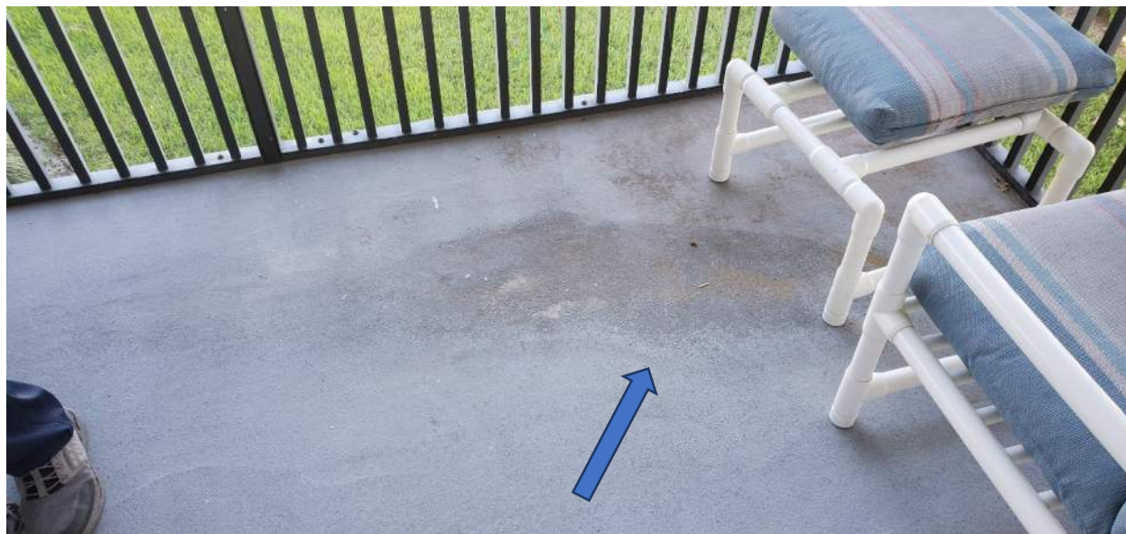
Example view of stained balcony floor coatings
