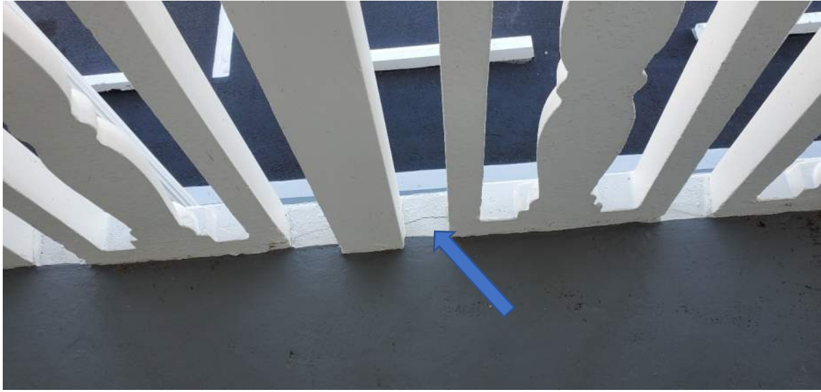
Example view of concrete walkway edge spalling
