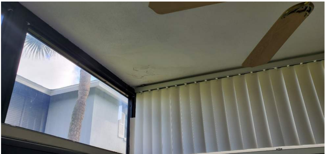
Example view of concrete slab ceiling spall
