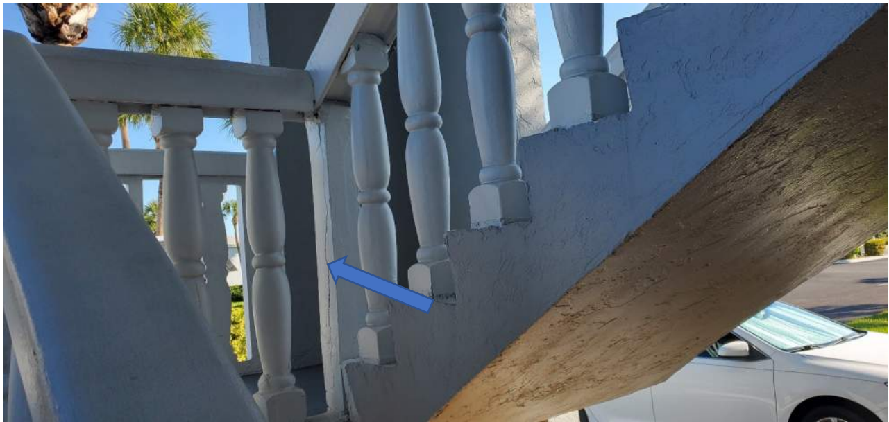
Example view of concrete walkway stair spalling
