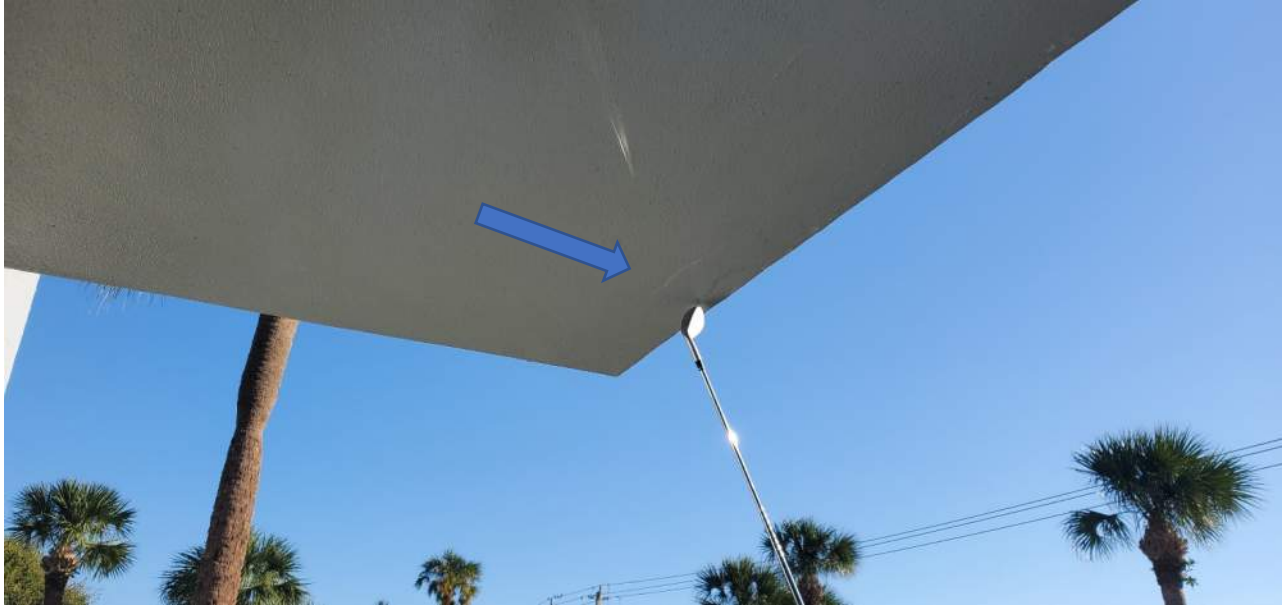
Example view of spalling concrete slab ceiling
