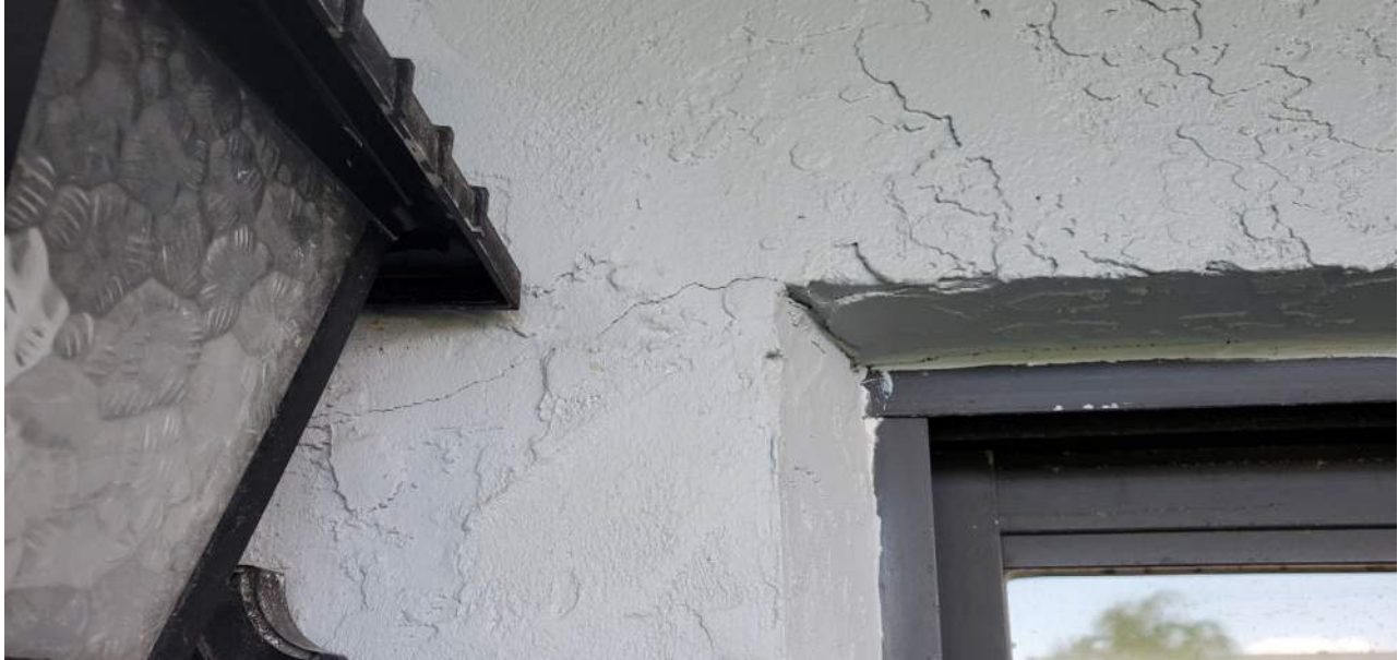
Example view of concrete wall cracks adjacent to sliding glass door header
