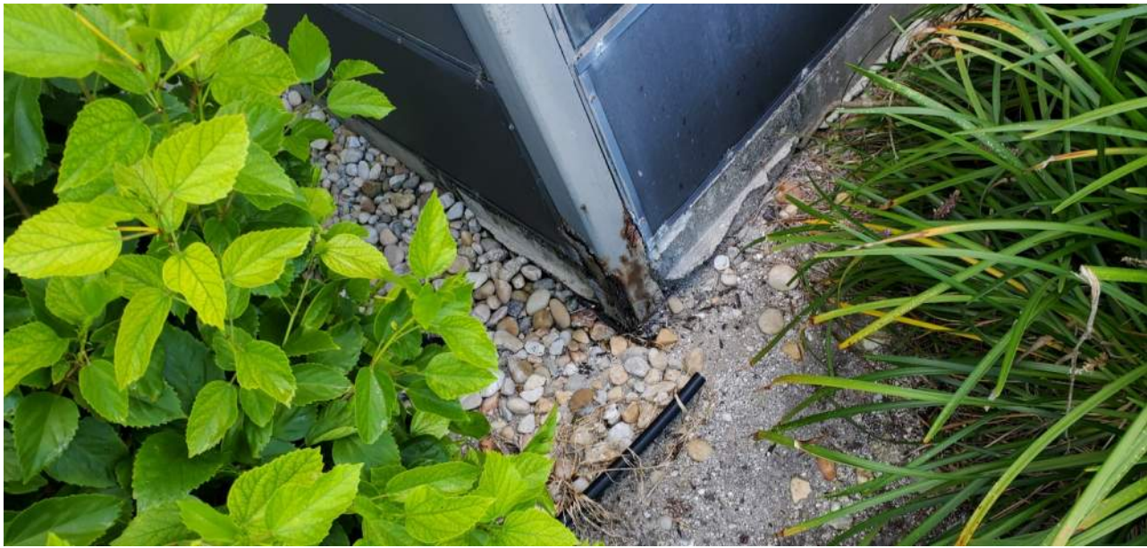
Example view of corroded corner column of screened porch
