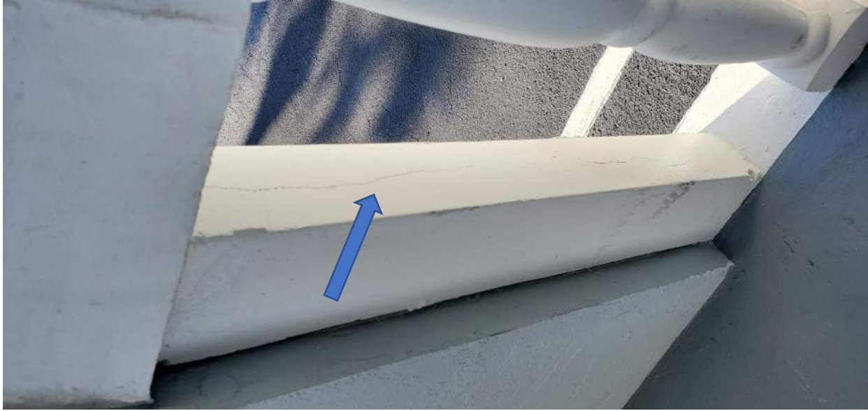
Example view of spalling concrete walkway railing picket
