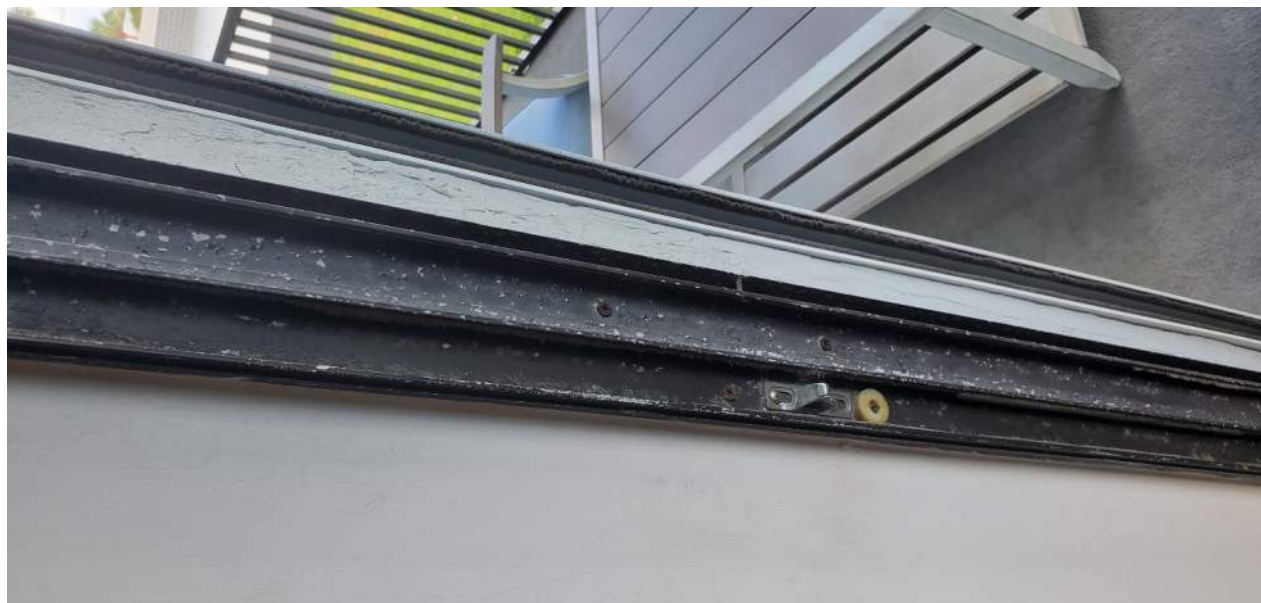
Example view of rusting and missing sliding door fasteners
