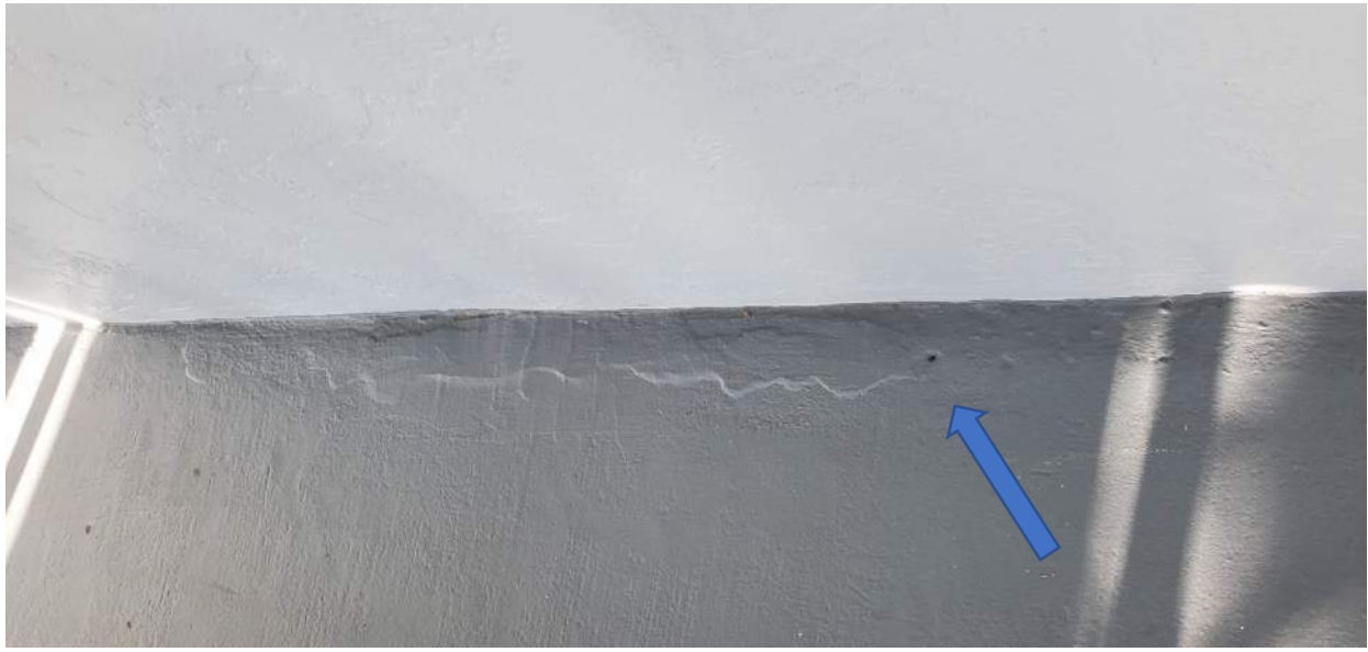
Example view of concrete walkway spalling and rust spots
