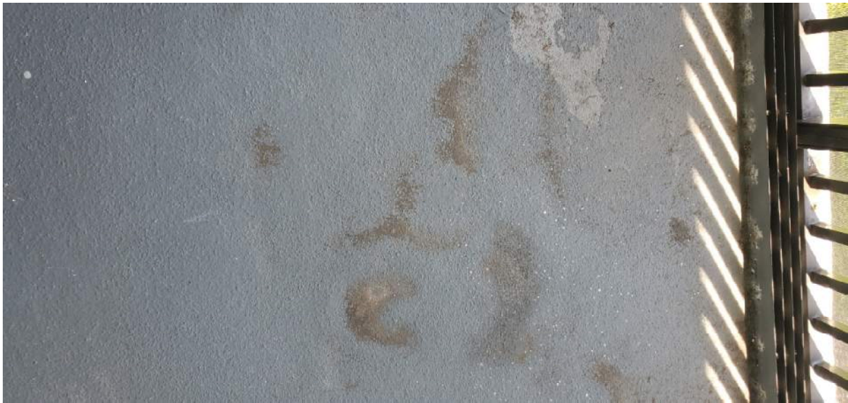
Example view of slab with bad coatings
