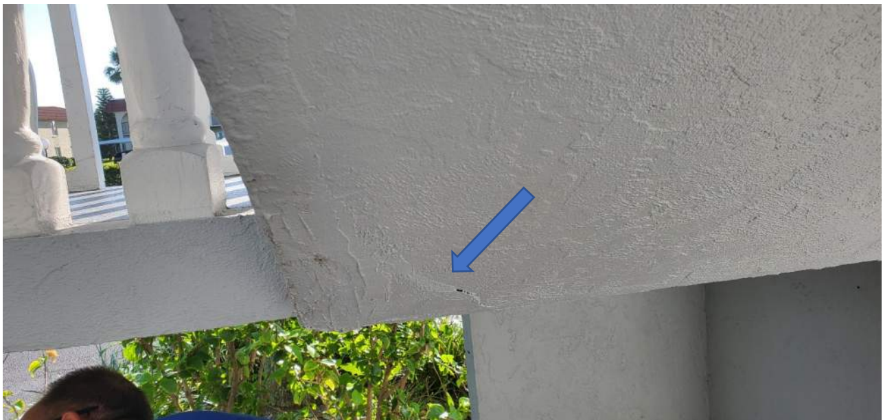
Example view of concrete stairs spalling
