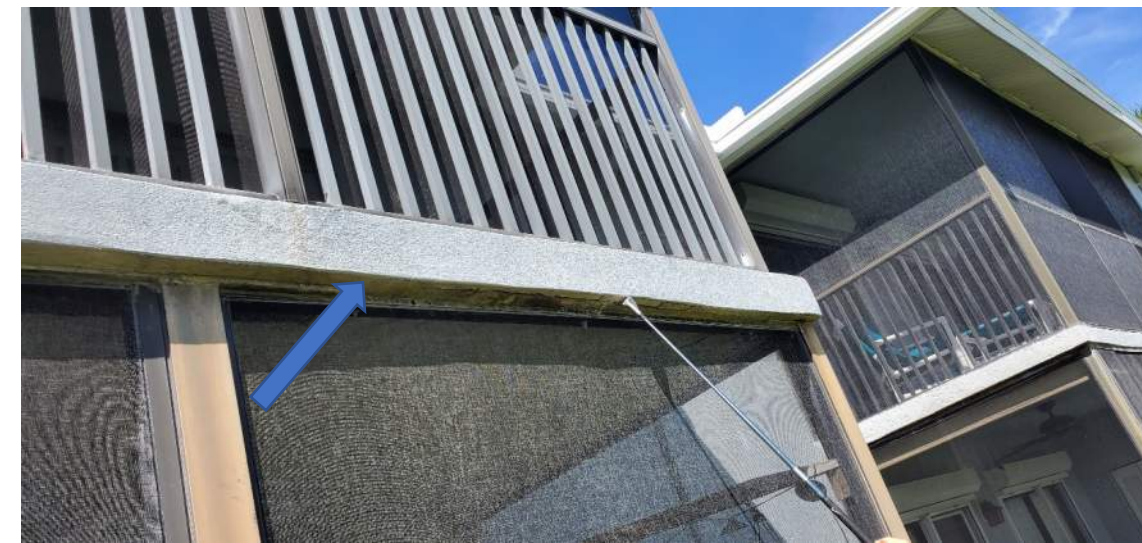
Example view of concrete beam spalling
