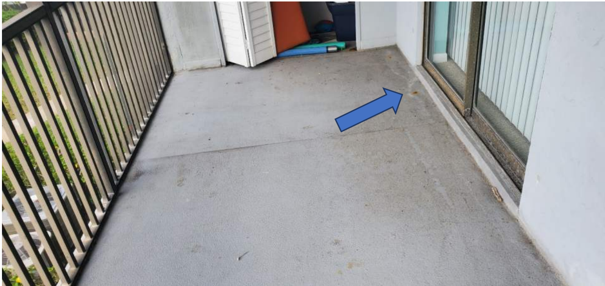
Example view of concrete spalling by the slider
